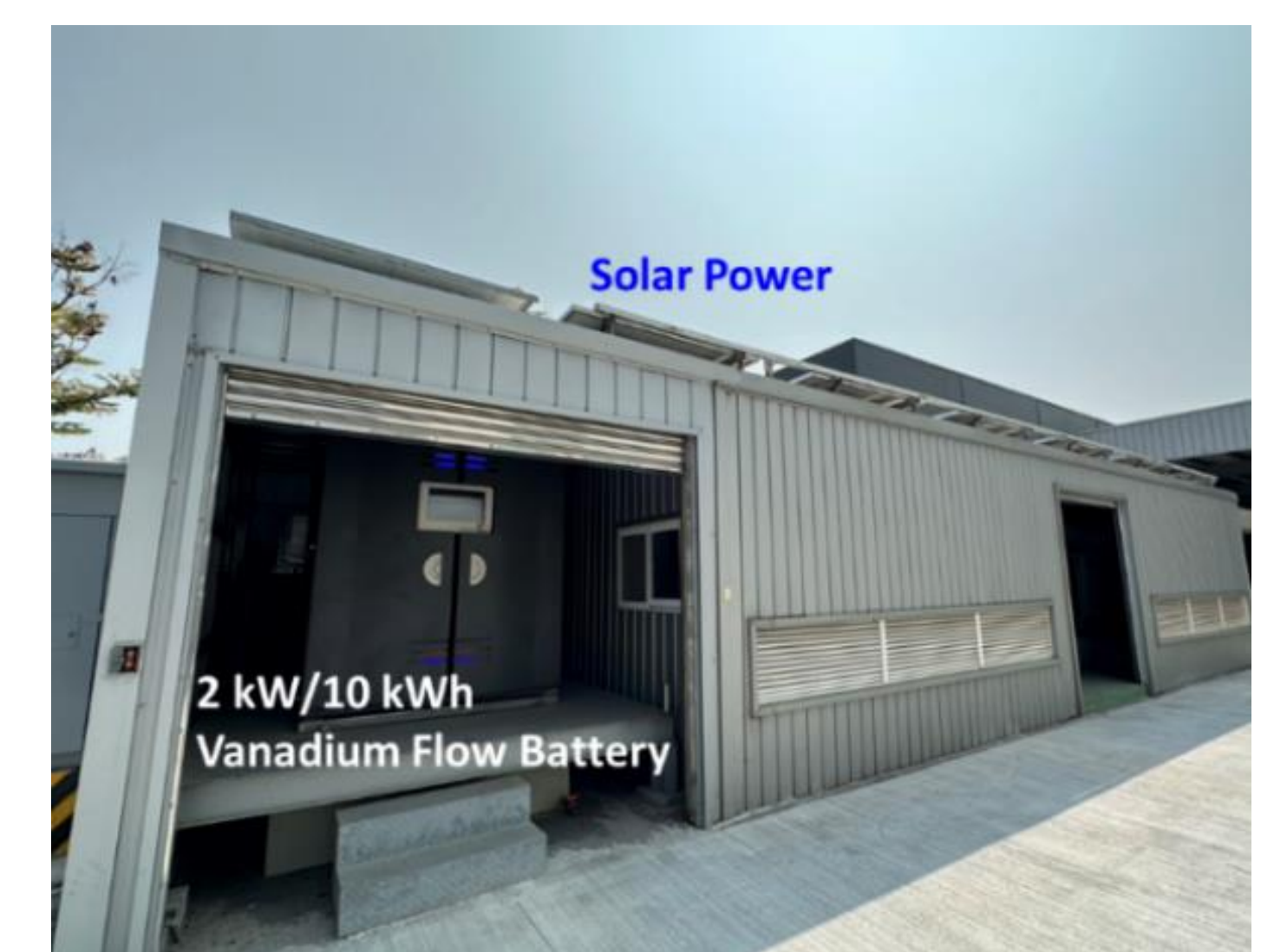
Figure 3. 2 kW/10 kWh vanadium flow battery system integrated with solar power.
